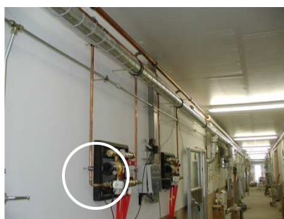
Fig. 14: Wrong - missing insulation at the supply line
